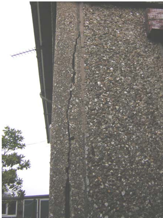
Photograph 2 – Vertical Cracking Of Corner Post
